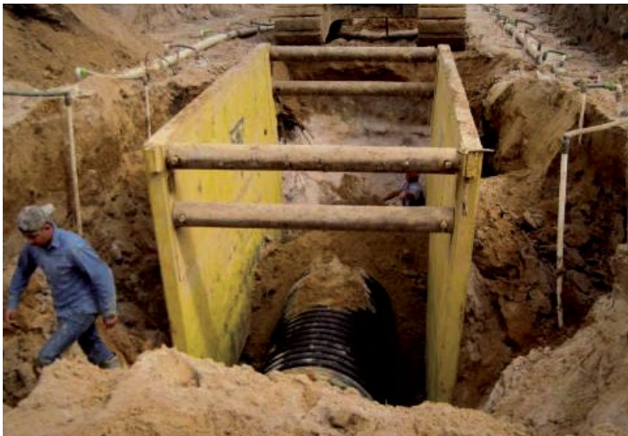
Safety versus proper installation 3.3 km of HDPE pipe ranging in size from 750mm to 1500mm failed on this project and had to be replaced
