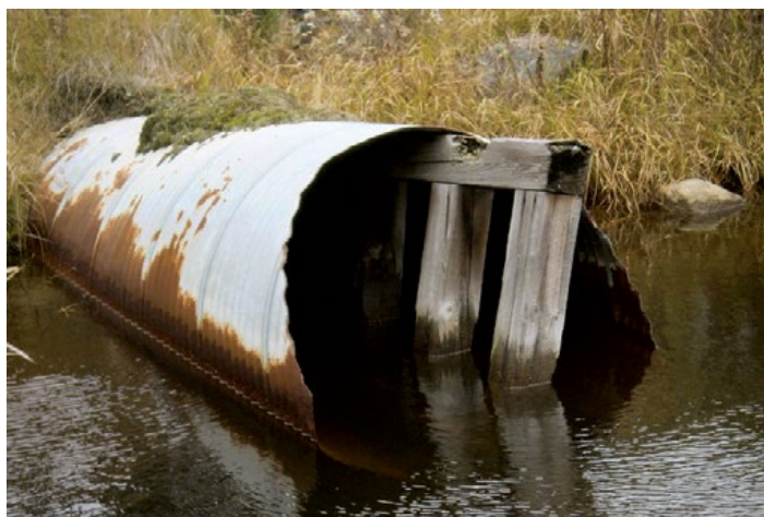
Deteriorated culverts under Trans Canada Highway
