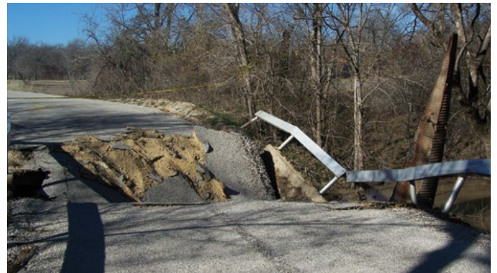
Crater caused by the corrugated steel pipe failure A section of the CSP is visible on the right hand side of the picture projecting vertically photo credit: John Dutschmann, Technical Resource Manager Hanson Pipe and Precast
