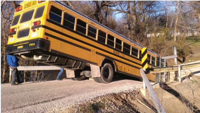
A school bus in a crater caused by a collapsed corrugated steel pipe photo credit: Dustin Hood
