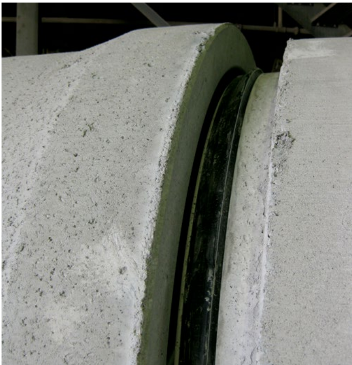
Concrete pipe joint with rubber gasket
