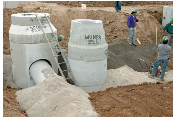
Reinforced concrete pipe, maintenance holes and catch basins for storm sewers, now underground
