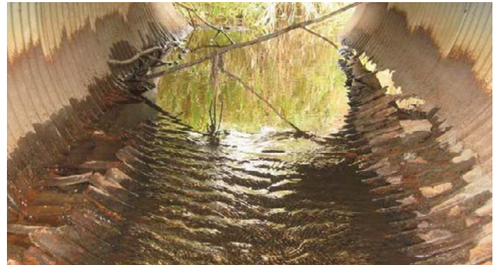
Rusted CSP culvert in service under busy Ontario highway
