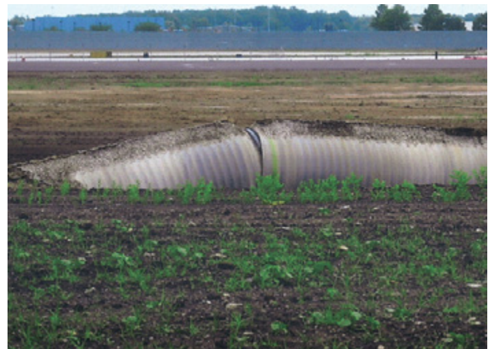
Columbus, Ohio Airport – polypropylene pipe floating out of ground
