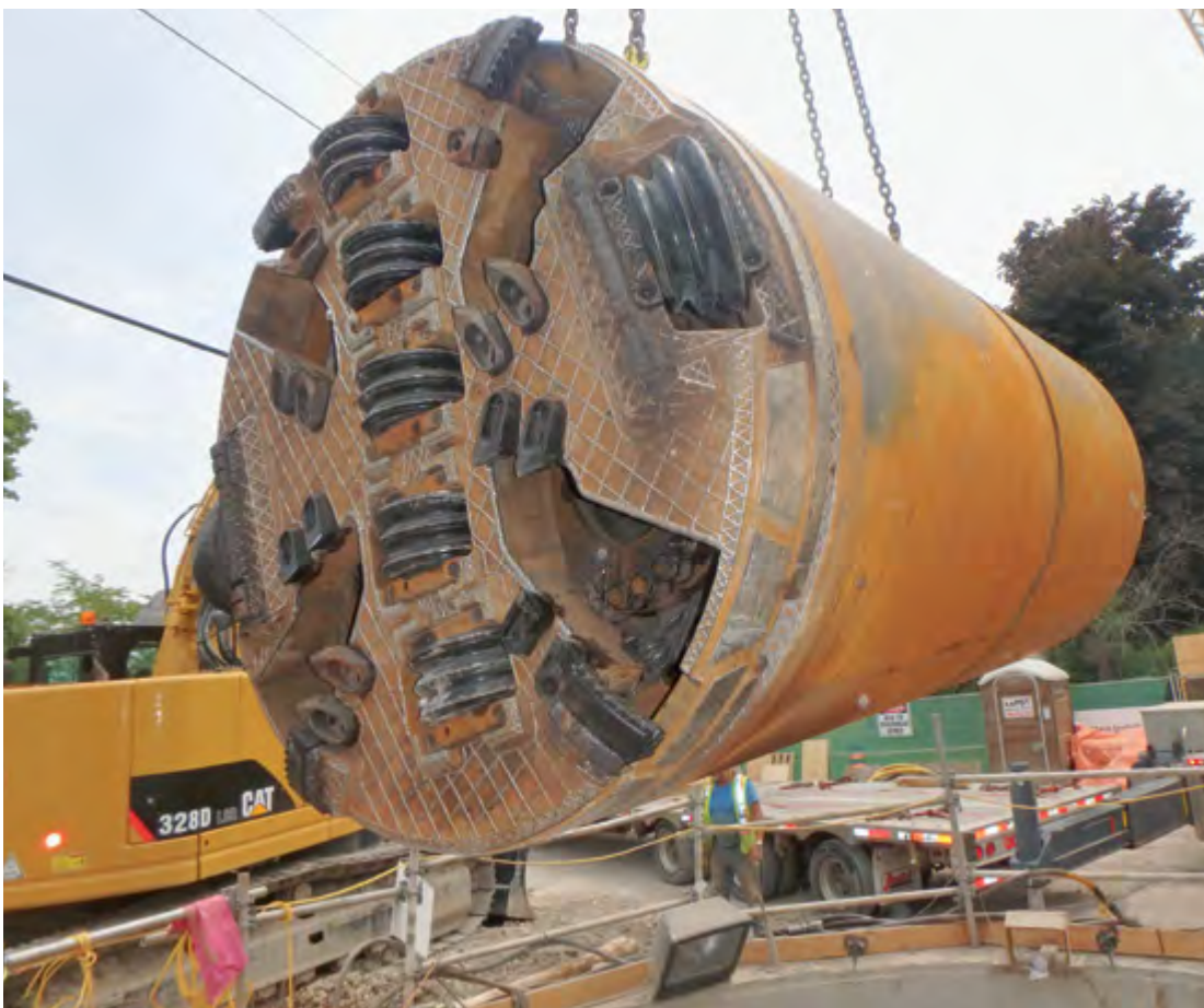
The project included nine microtunneling drives (eight curved) ranging in length from 180 to 626 m (590 to 2,053 ft), with seven of the drives completed in rock.
