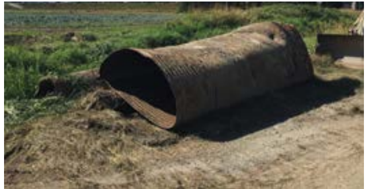
Severely corroded corrugated steel pipe Photos: The Langley Concrete Group of Companies
